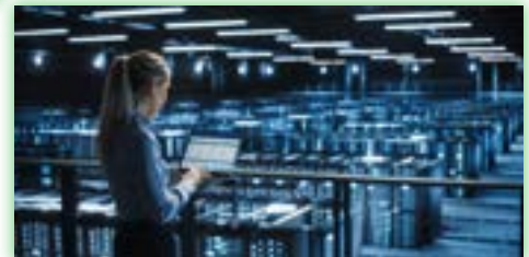
Micro Data Center and Server Room
